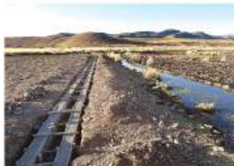
Construction of more efficient irrigation canal in The Altiplano. (Photo Dirk Hoffmann)
